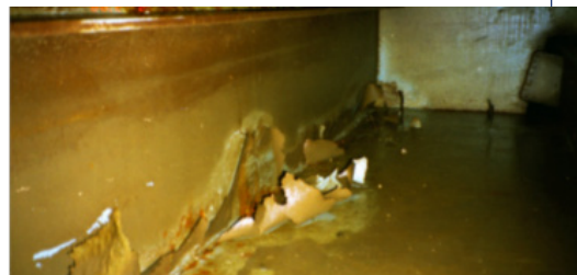
Corrosion takes its toll
